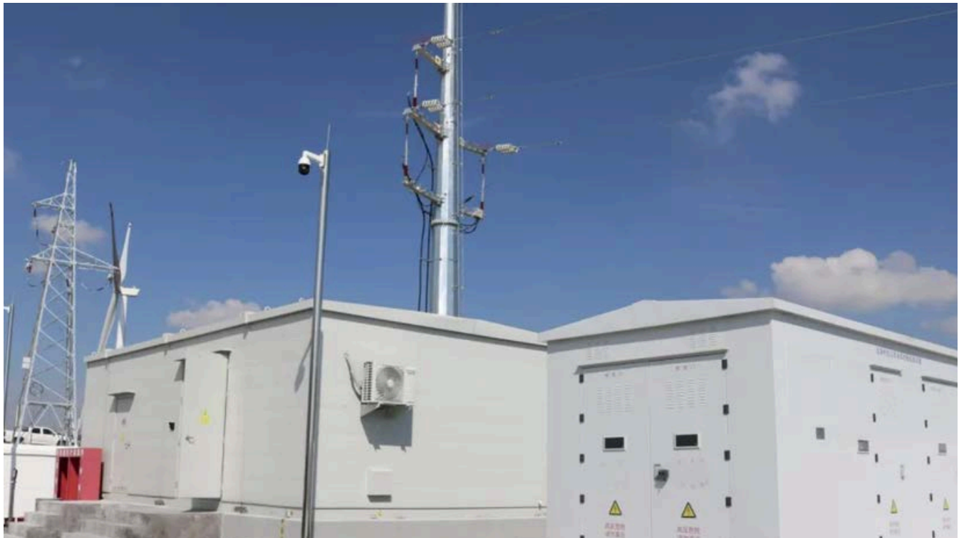
Project electrical control room
